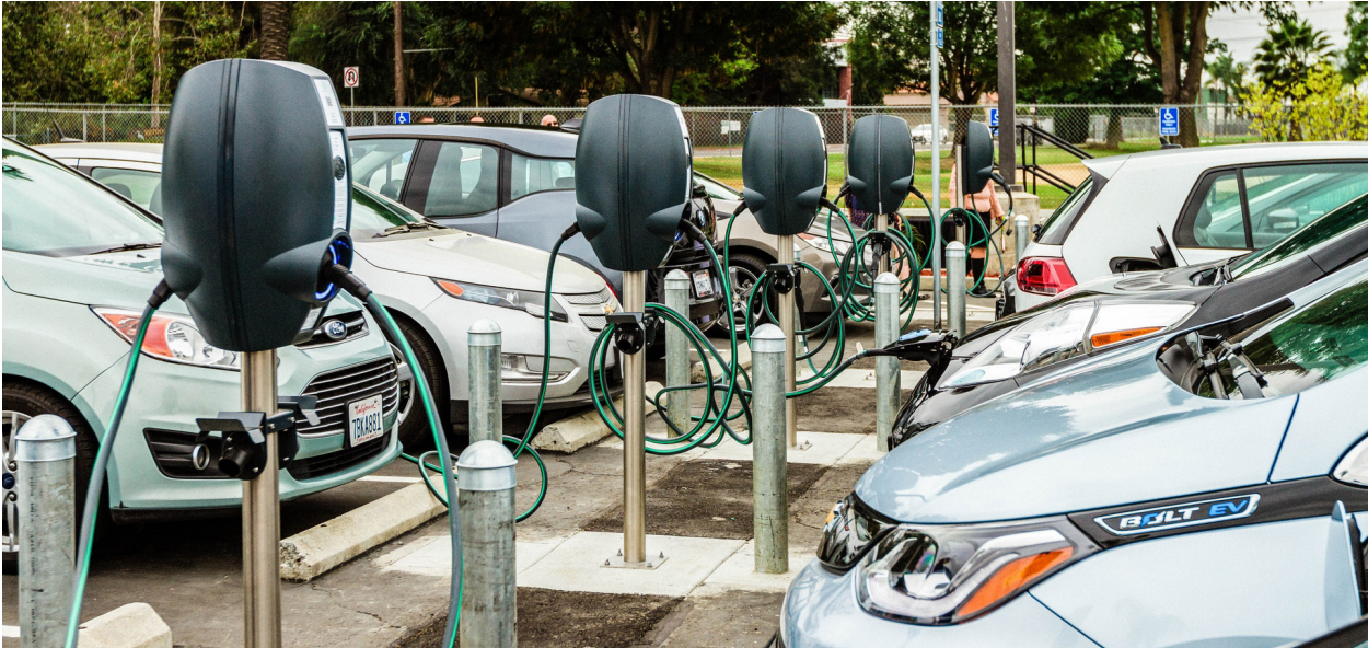
Charging stations in South El Monte. To date, SCE's Charge Ready program, with its customers and partners, has installed more than 1,000 EV charging ports at more than 60 different sites. Photo: Maria Hedrick.
